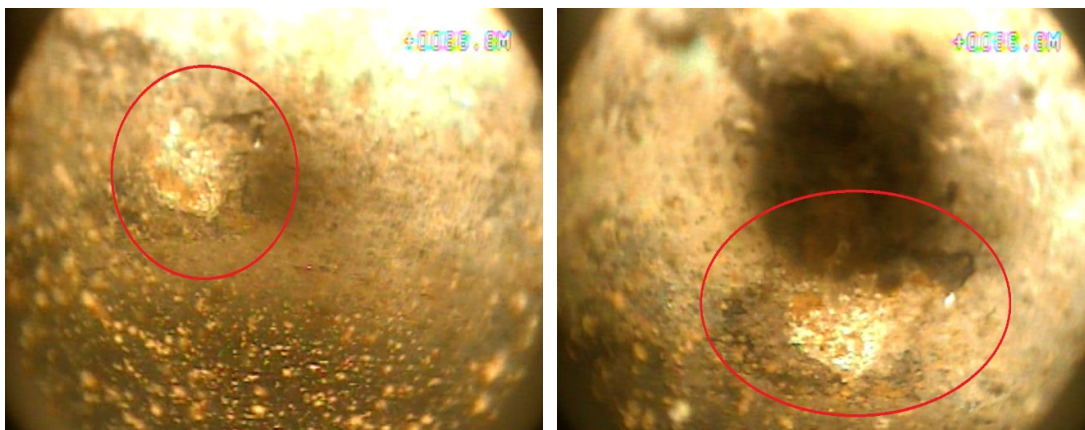
Significant corrosion / hole noted through mild steel casing wall at 86.80m.
