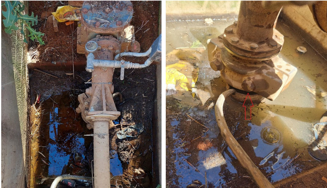
Unsealed headworks as viewed from surface.
