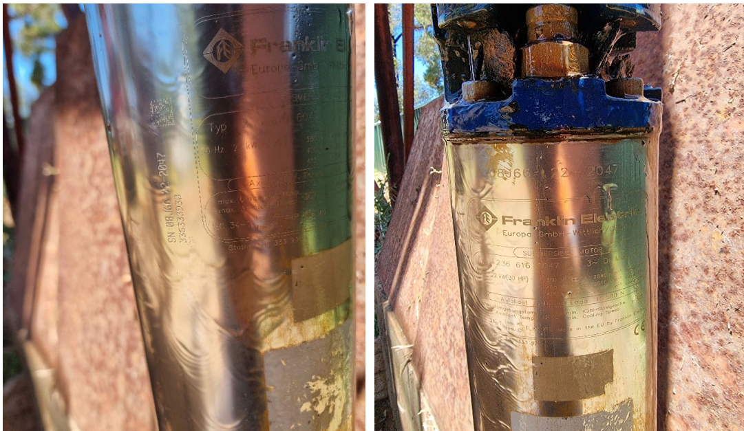
Identification plates as noted on submersible pump.
